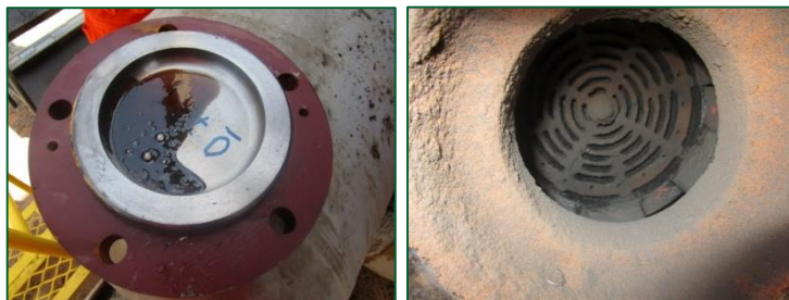
Figure 3. Compressor valve failure showing contaminants in the compressor
