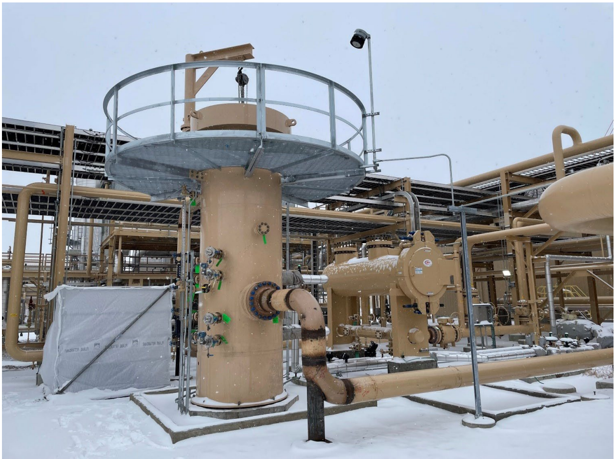
Figure 4 – Transcend Solutions vertical residue gas coalescer (left foreground) and previous horizontal filter coalescer (right background). Scaffold tent to the left of the vertical coalescer is the enclosed shelter for the test apparatus.
